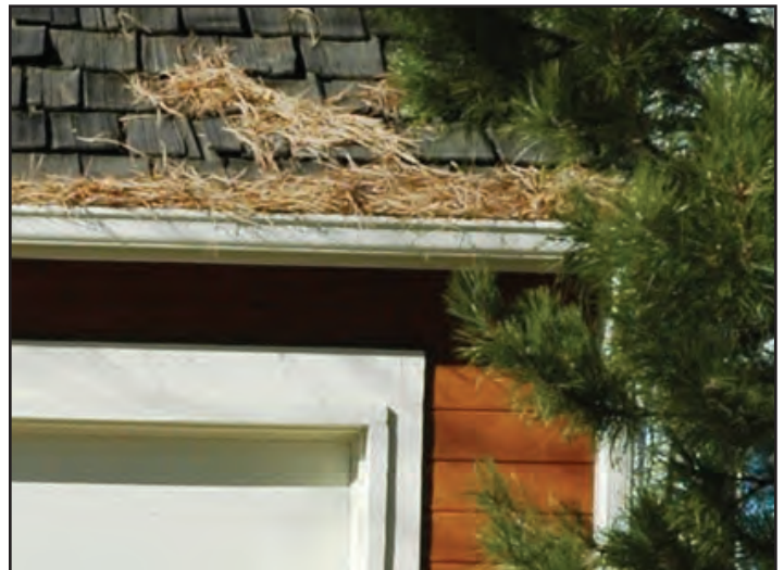
This roof is extra vulnerable to embers because needles have accumulated in the gutter below an aging wood-shake shingle roofing assembly. Photo by South Metro Fire Rescue.
