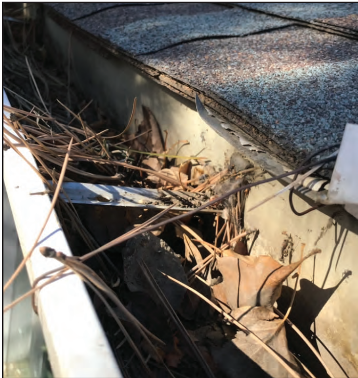
Dead needles and leaves in this gutter are easy fuel for spot fires caused by embers. Photo by South Metro Fire Rescue.
