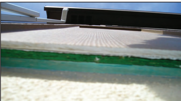
A gap between siding and the foundation at the base of a wall. Photo by Colorado Springs Fire Department.
