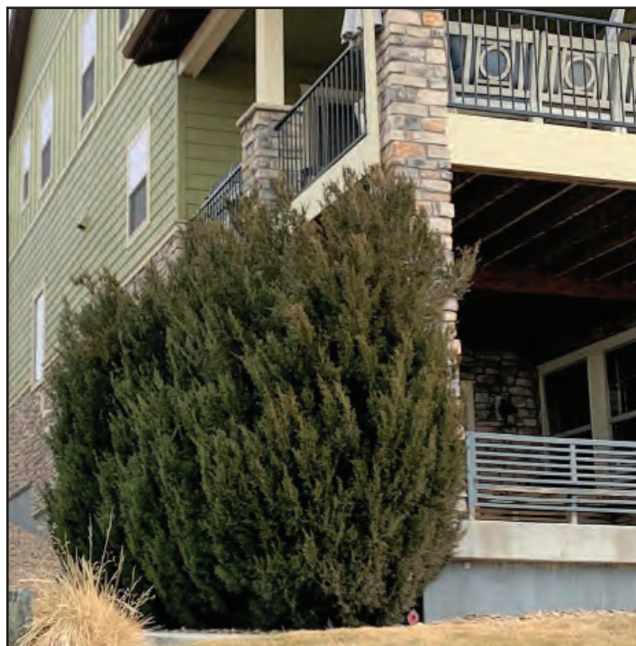
These junipers are too close to the home. In addition to releasing radiant heat, their convective heat could pool under the deck. Photo by South Metro Fire Rescue.
