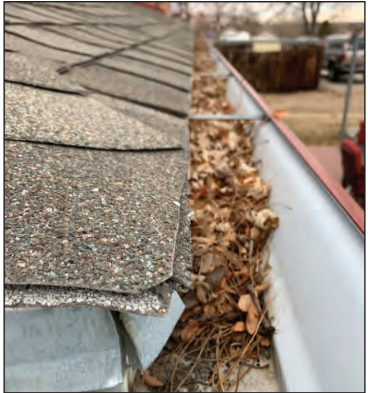
If these dead leaves catch fire, heat may flow under the asphalt shingles igniting the roof assembly and attic. A screen, such as one in the photo at right, prevents combustible debris from accumulating in gutters. Photos by South Metro Fire Rescue.
