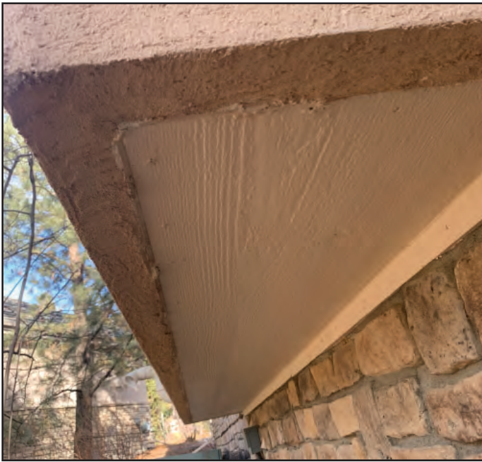
This projection is less vulnerable to pooling convective heat because it is protected by a layer of wood. Photo by South Metro Fire Rescue.
